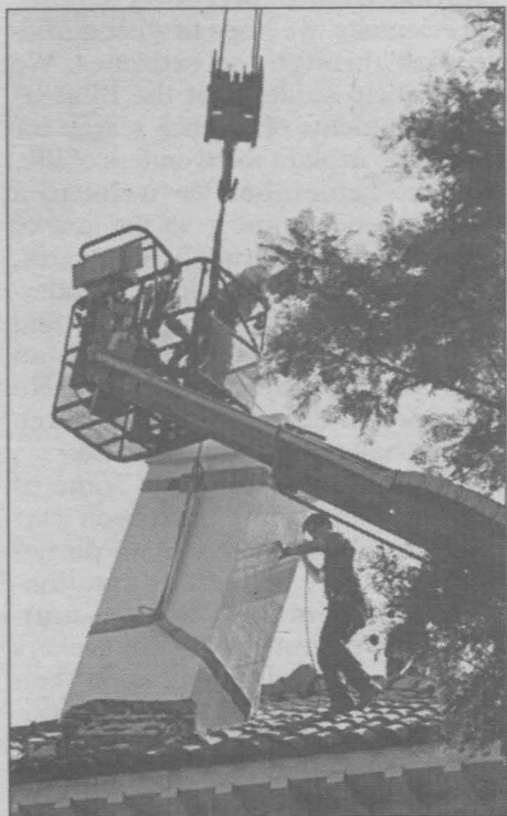
AMBASSADOR HALL —A quake-damaged chimney tilting 15 degrees was removed from roof. [Photo by Hal Finch]
